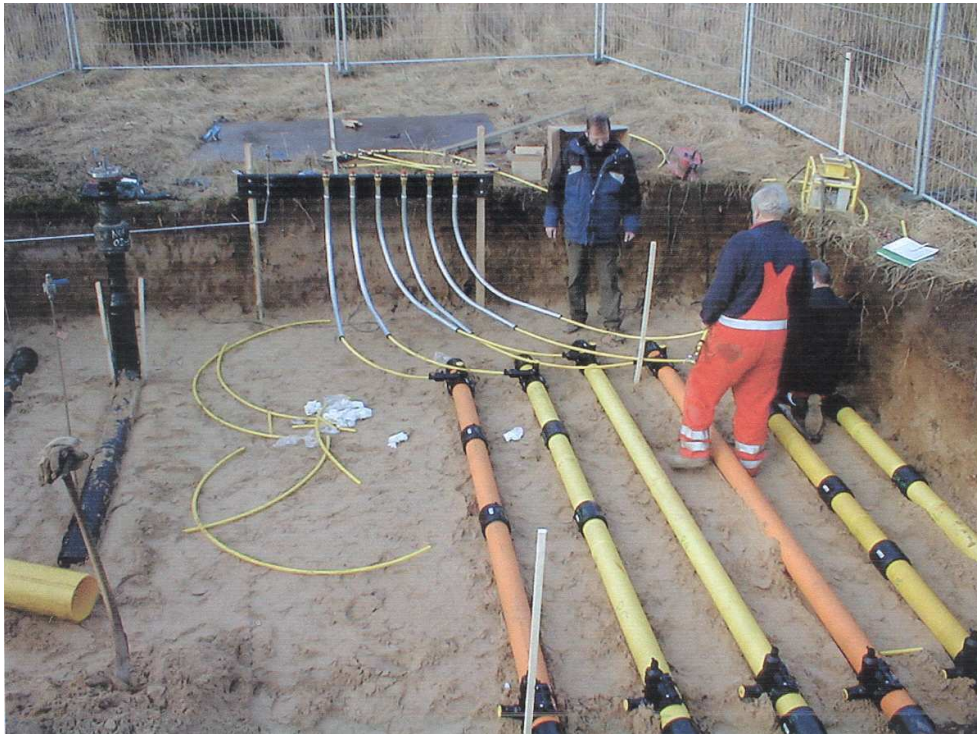
Figure 1: The photo shows laying of the test pipes. The two black pipes to the left are 19 bar steel distribution pipes. The other pipes are new and second-hand pipes from the Danish and Swedish gas grid.
